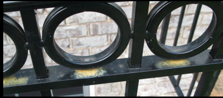
Products that are not coated pre-assembly are more likely to rust.
